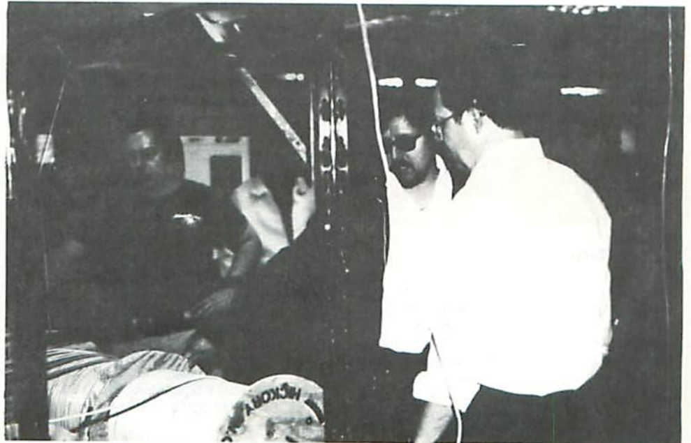
Installing fiber-optics cable in Marlboro are: (l. to r.) Jim Burgess, data communication technician; Bob Holt, principal fiber optics design engineer; and Roy Evans, CSSE senior maintainability engineer.
