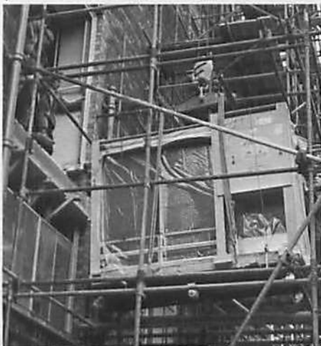
Via specially erected scaffolding, and with a professional ease that amazes the man-in-the-street, removal men deliver Manchester University's new DEC PDP-10 computer through a second-floor window.
