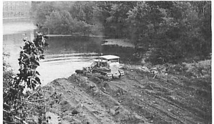
Increasing Parking Facilities — Bulldozers are at work filling part of the mill pond near Digital's Thompson St. entrance to expand our parking area.
