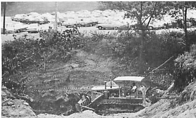
Our contractor for the parking lot project is A. Amorello & Sons, Inc. of Worcester. Here, one of the bulldozers clears space near our present parking facility.
