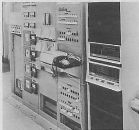
Remote PDP-8/S controlled pumping station along Interprovincial's pipeline is linked to station controls by monitoring and control equipment designed by Computer Special Systems.
